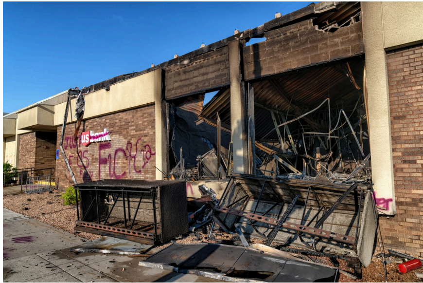
Figure 2.1.2: Building with fire damage.
