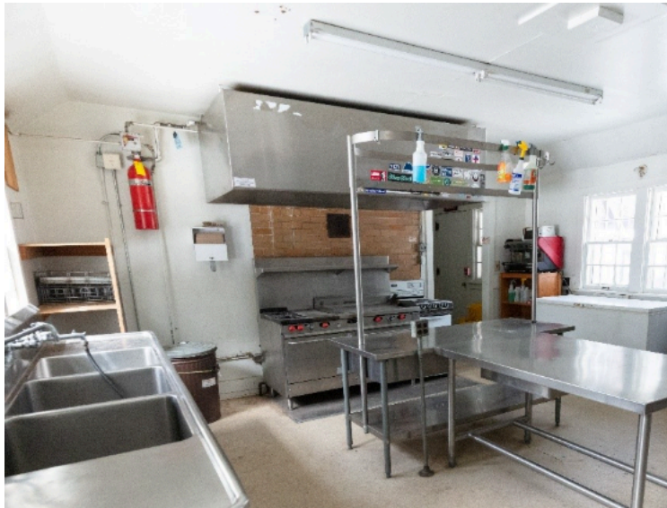
Figure 7.2.2: Extinguisher in a commercial kitchen.
