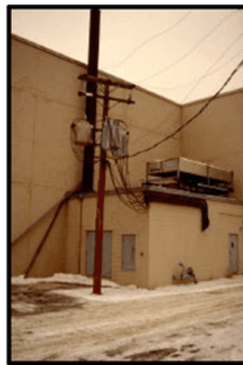
Service Drop Line
