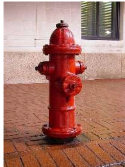
Figure 2.2.7: Downtown Charlottesville Fire Hydrant by Ben Schumin is licensed under CC BY-SA 2.5
