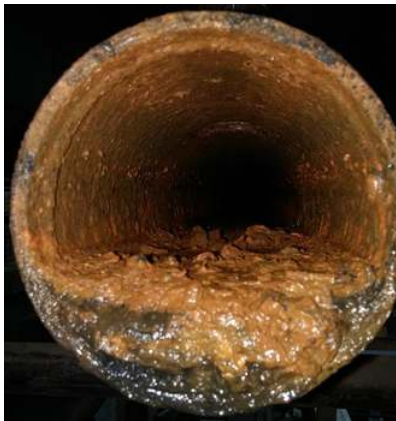
Figure Chapter 11.5:Pipe with corrosion . (Copyright: Image by Mr pantswearer is licensed under CC BY-SA 4.0 .)
