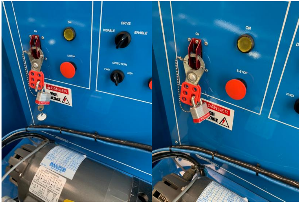
Figure 7.C.3: LOTO, unsafe and safe condition. (Source; William Oneil-Chaffey College)
