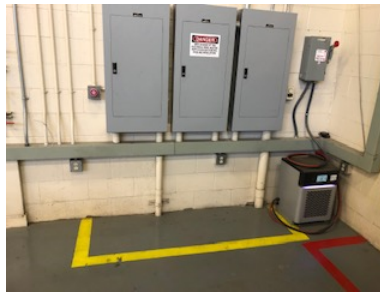
Figure 9.A.4: Electrical Panel and Safety Switch. (Source; Greg Ling-Long Beach City College)
