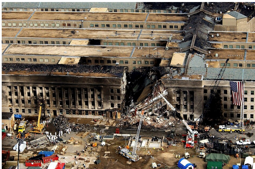
Figure 7.3.1: A photograph of the damage to the Pentagon caused by the 9/11 attacks. (CC0 1.0; TSGT CEDRIC H. RUDISILL, USAF via Wikimedia Commons). Detailed Description of Figure 7.3.1.
