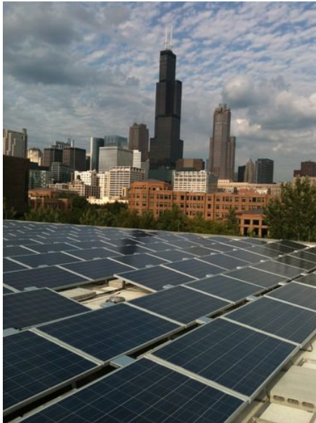
Figure 12.3.4: Rooftop Solar Installations Rooftop solar installation on Douglas Hall at the University of Illinois at Chicago has no effect on land resources, while producing electricity with zero emissions. Source: Office of Sustainability, UIC
