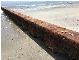
Figure 1.1.2: Port Royal, South Carolina oxidation of iron. Image courtesy of Elizabeth R. Gordon.
