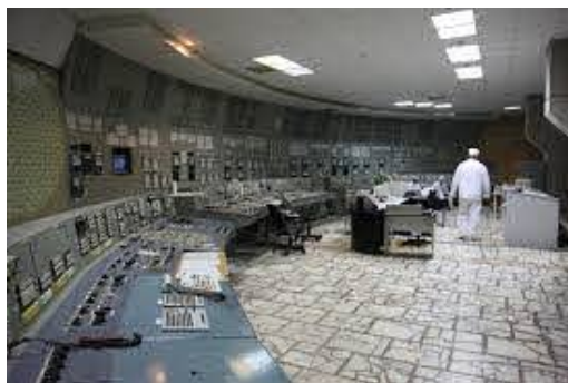
Figure 5.6.6.2: Interior view of the control room of Chernobyl Nuclear Power Plant unit 3. Over 3,000 people continue to work at Chernobyl to monitor nuclear fuel and carry out the decommissioning of the facility. ( www.iaea.org/NewsCenter/Multi...bank/index.js )
