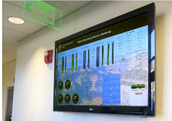
Figure 3.5: Real-time building energy monitoring example.
